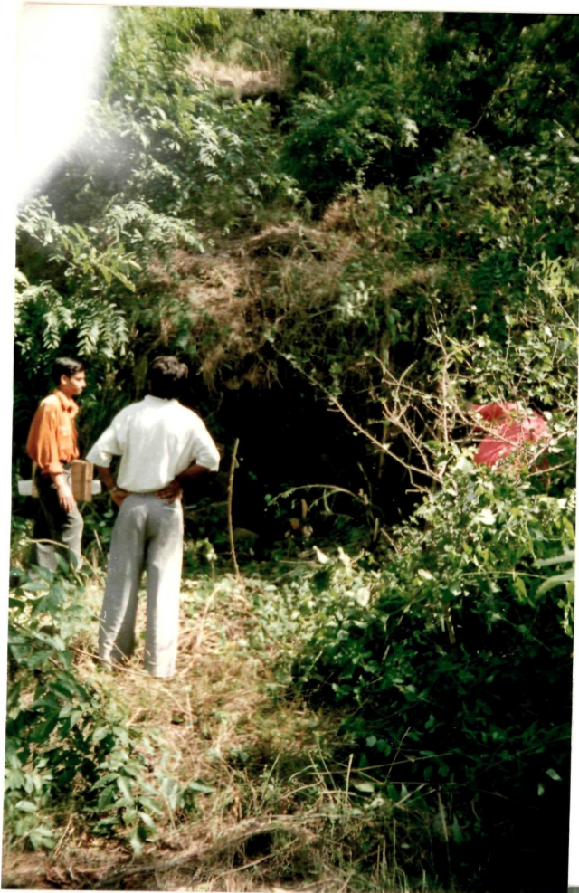
PLATE NO 47 DAMAGED STRUCTURAL OF UNDERGROUND TUNNEL
