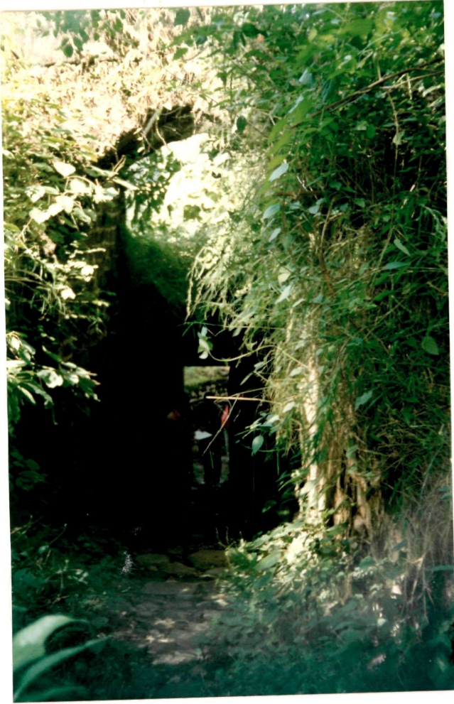
PLATE NO 51 RUINED STRUCTURE OF WESTERN DARWAZA NO-I HAVING 6.00 MTRS HEIGHT SIZE
